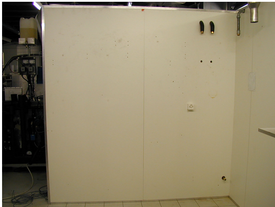
Figure 1: Floor installation area. A 25 cm grid drawn on the floor gives an indication of the space requirement from that photograph alone.
