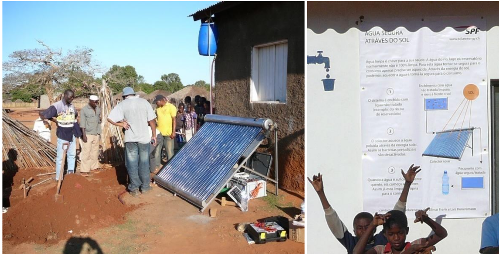
Fig. 11: One of four different system-implementation sites (here in rural Mocambique). Left picture: a local team is trained for the installation, maintenance and operation. Right picture, background: information campaign about water-hygiene and the water disinfection system.
