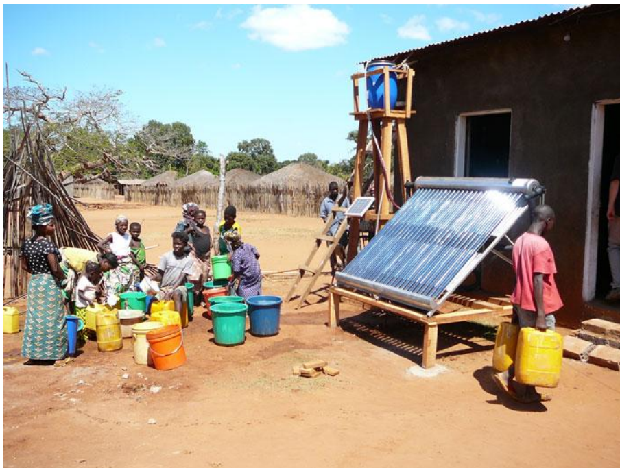
Fig. 1: The solar thermal water disinfection system installed at a testing site in rural Mocambique.
